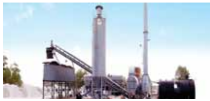
100 metric ton per hour capacity drum plant at Puchong, Selangor
