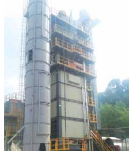
180 metric ton per hour capacity batch plant at Ulu Langat, Selangor
