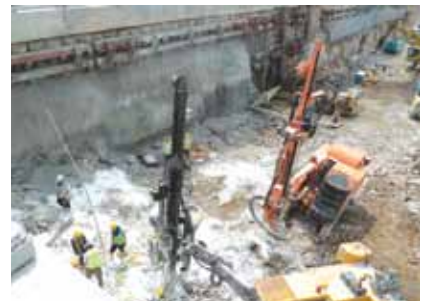
Excavation works with controlled blasting to construct an underground station for MRT.
