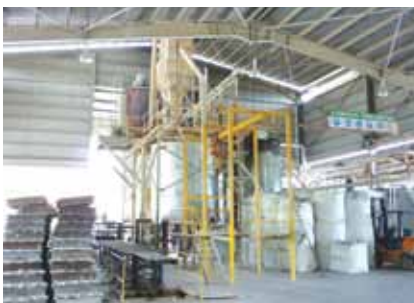
Tankage used in the production process
