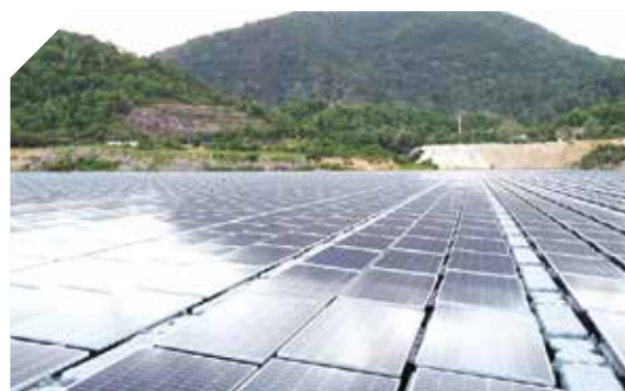
Solar Power Plant in Pantai Remis, Perak
