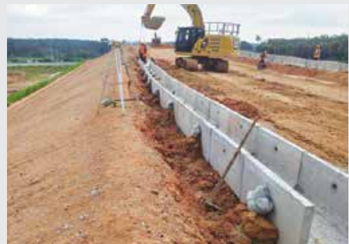
Civil engineering works for the Electrified Double Track from Gemas to Johor Bahru
