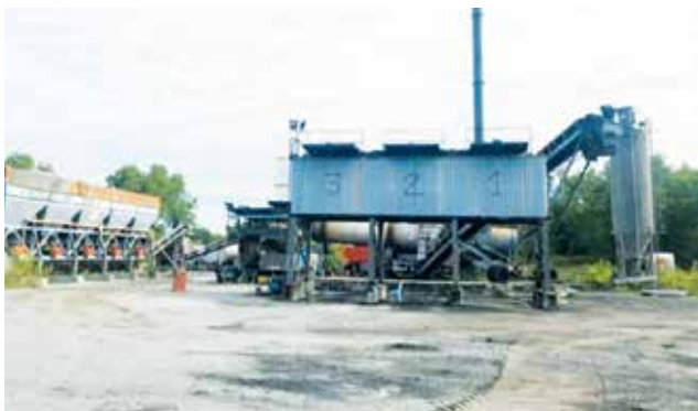
180 metric ton per hour capacity drum mix plant at Saujana Puchong, Selangor
