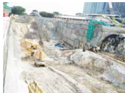
Excavation works with controlled blasting to construct an underground station for the MRT 2 project
